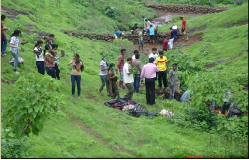
Construction of small bunds across rivulets through shramdan at one of Hariyali's projects at Bhavale, Thane Dist, to arrest water.
