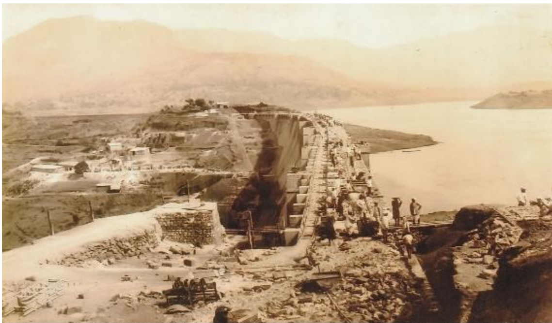
23 - Dam at the end of May 1924 Height 270 Ft, above River Bed Cross View from North Bank
