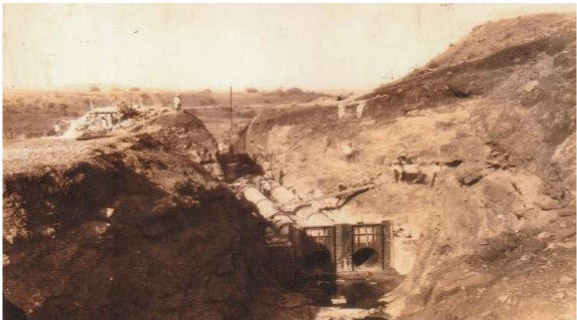
71 - The Third Set of Steel Outlet Pipes at 150 Ft. Above River Bed. View from the Up Stream - May 1919
