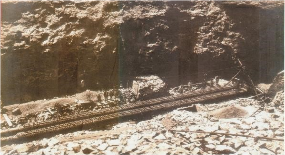
46 - The Lowest Steel outlet pipes two off 3 die at 50 ft. above River Bed Showing Steel Reinforcement For cement Concrete, casing of Up Stream End - March 1916
