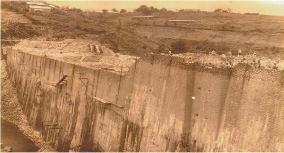
60 - Dam in May 1918 Average 1918 Height 135 Ft. Above River Bed Up Stream face from the South Bank
