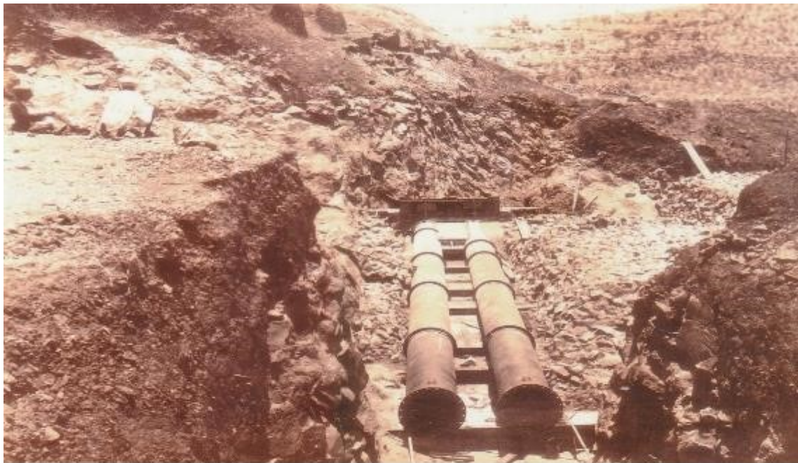
70 - The Third Set of Steel Outlet Pipes at 150 Ft. Above River Bed Showing the laying Arrangement.
