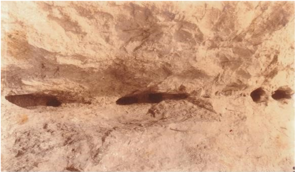
76 - Pockets in Crack in Rock Foundation on Southern Bank Beyond 150 Ft. Outlet - 1919
