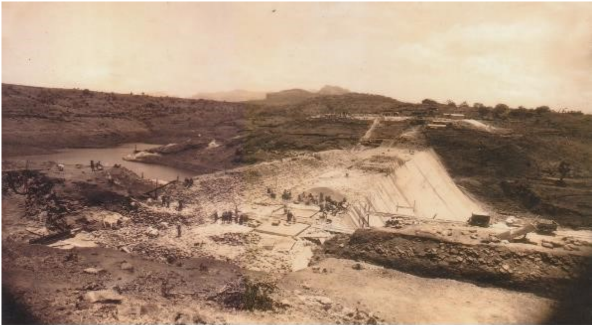
50 - Dam in March 1916 Highest Part 110 Ft. Above River Bed Cross View of the Dam from Left Bank
