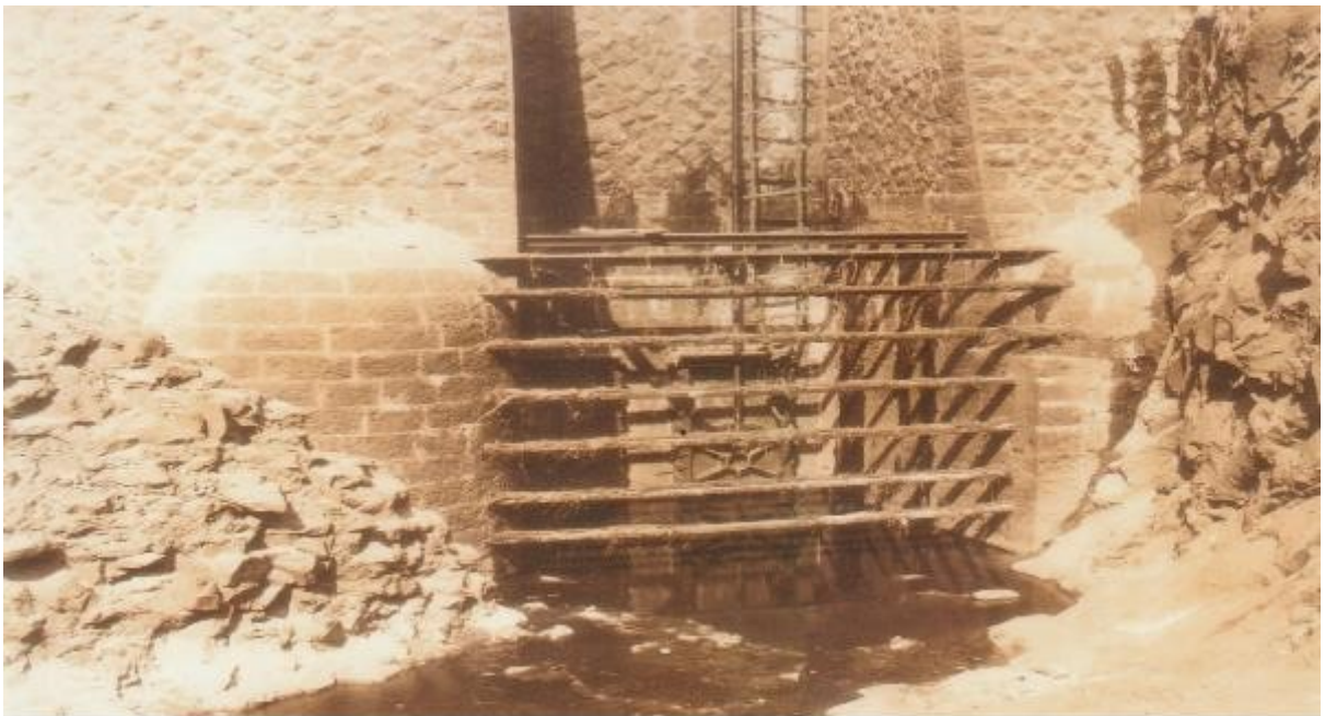
63 - The Second Set of Steel Outlet Pipes at 100 Ft, Above River Bed Showing the complete Arrangement of casing - ( May 1918)
